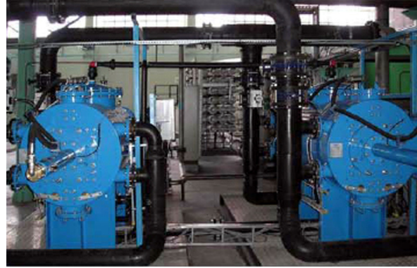
Prefiltration to RO system, demineralized water. Steel Mill, Ukraine
