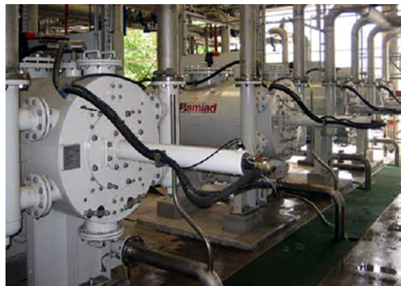
Pre-filtration for RO with 2 lines of 200 m 3 /h at 3 \mu . 4 filter units for 100% security. Raw city water with quality with SDI <2. Petrochemical industry. France
