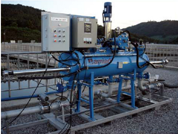
River water for industrial purposes. TSS removal from 2.3 mg/l to 3 mg/l. 28 m 3 /h. Korea
