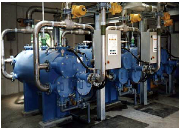
Backwash water from sand filters at a WTP to remove cryptosporidium, enabling 10 MI/day to be reclaimed drinking purposes. United Kingdom
