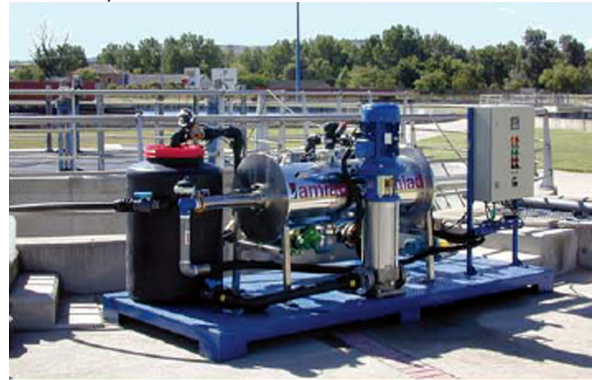
Test unit. Pilot objectives are to reduce TSS & NTU to meet "California Regulations" in effluent tertiary treatment
