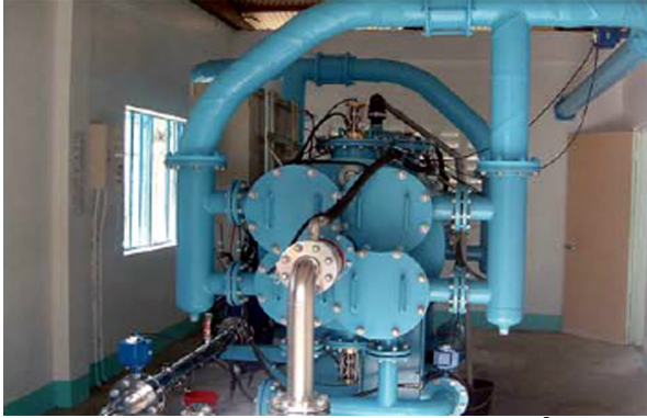
Surface water used for drinking water. 120 m 3 /h 3μ. Mindanao – Philippines
